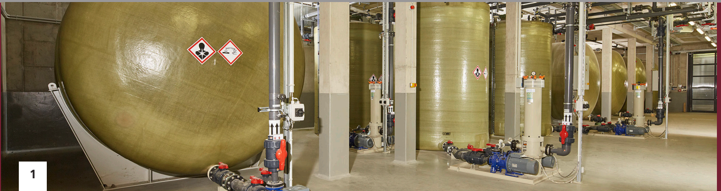
1 Organic redox flow batteries, a technology to store large quantities of energy from renewable sources. © Fraunhofer ICT
